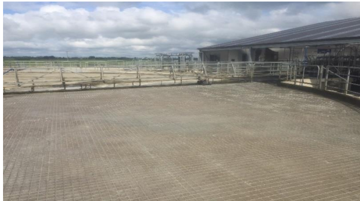
Concrete grooving close to the entry to the shed to help alleviate a slippery yard; thanks to Doug from 'Cow Yard Grooving'
